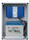
24V ups back up battery for extended power outages from 2 days to 2 weeks.
