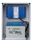
24V ups back up battery for extended power outages from 2 days to 2 weeks.
